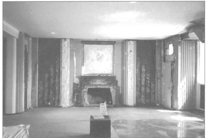
Original fireplace, fluted pilasters and mosaics after being uncovered. Note damaged/painted mosaics...
