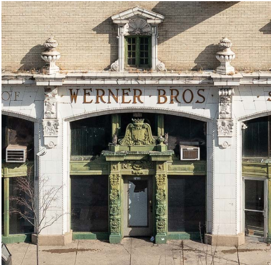
Werner Brothers Storage Warehouse, 1921, George S. Kingsley, 7613 N. Paulina Street. A 2023 Chicago 7 Most Endangered. Photo credit: Serhii Chrukky
